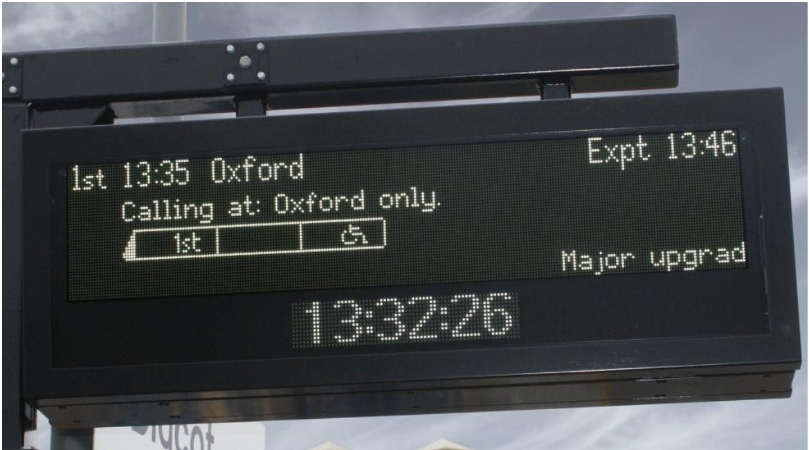
New platform Customer Information Screens
